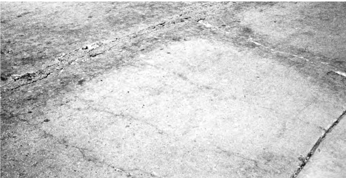
◀ Closely spaced, hairline transverse cracks. Indicates slab is broken and in need of replacement.
