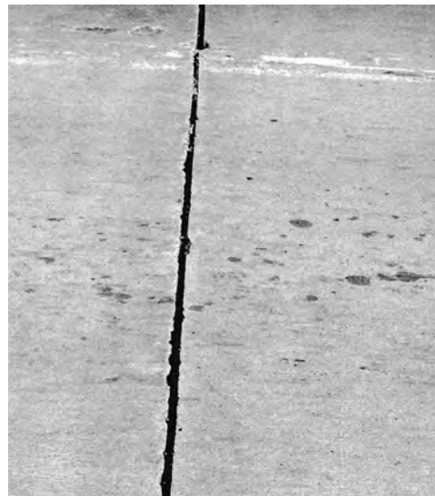
▲ Partial loss of joint sealant.
