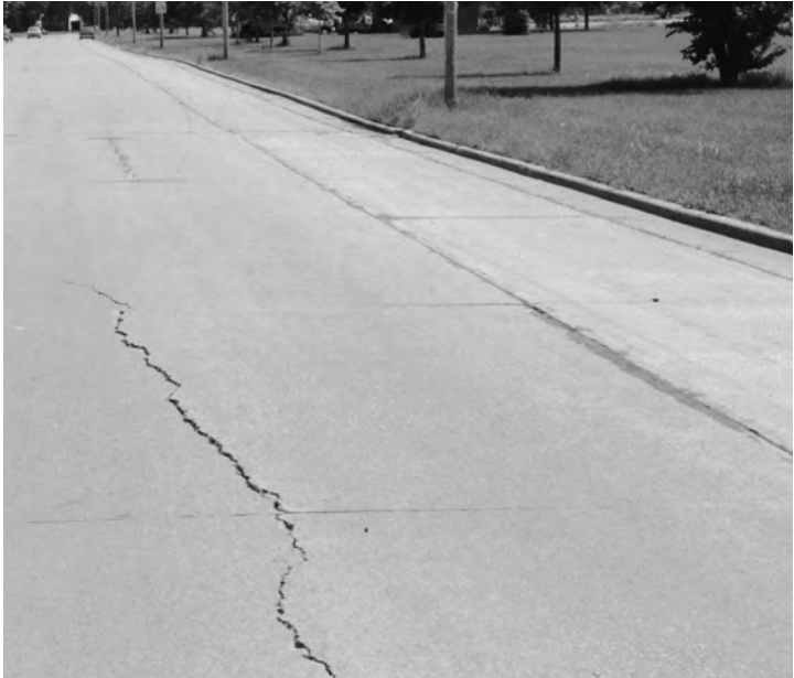
► Settlement caused meander crack with faulting.
