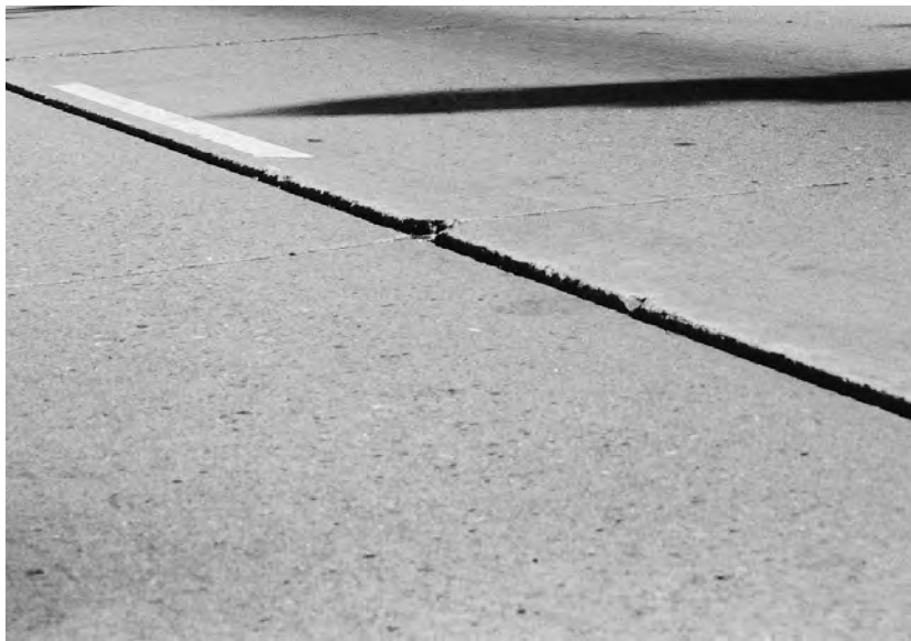
▲ Faulted longitudinal joint (over 1/2") with slight edge spalling.
