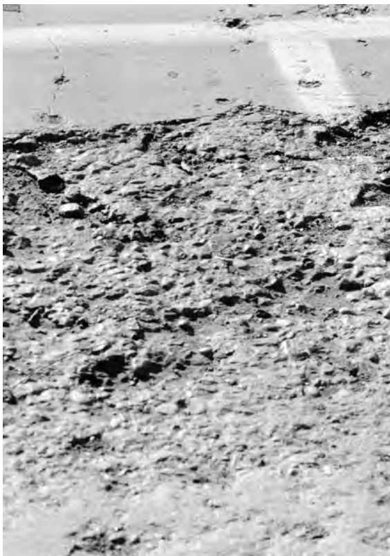
▲ Severe scaling over extensive areas. Patching or overlay needed.
