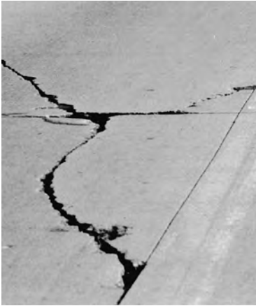
▼ Corner crack with spalling.
