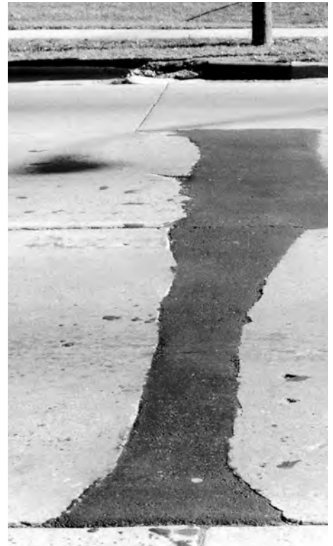
Patching in ▼ fair condition.
