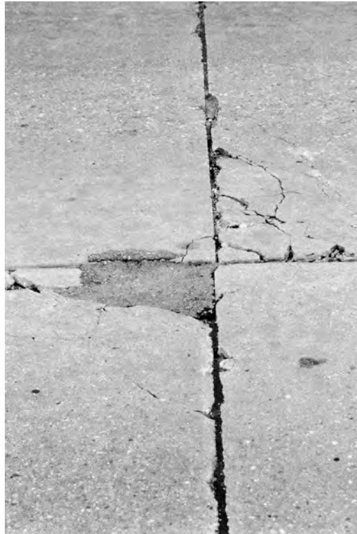
▶ Broken corner pieces. Some joint spalling.
