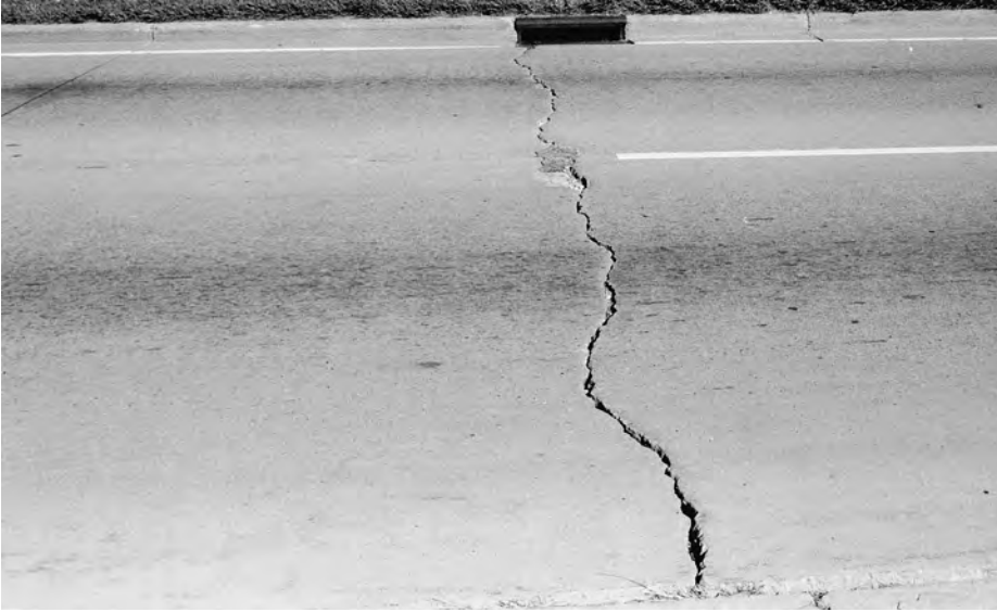
◀ Transverse, open crack.
