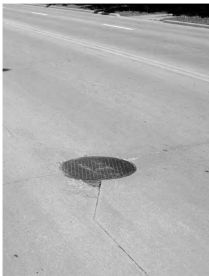
▶ Isolated spall at manhole.
