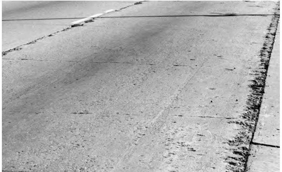
► Spalling along longitudinal joints.
