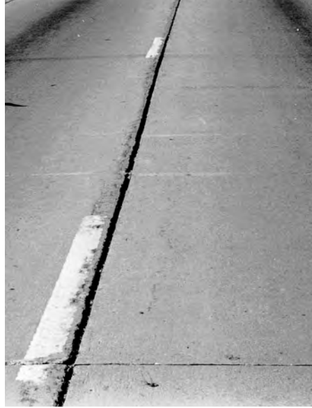
▲ Joint open about 1/2".
