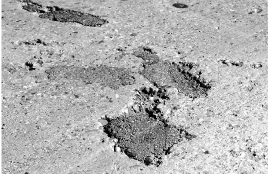
► Small surface spalls that have been patched.
