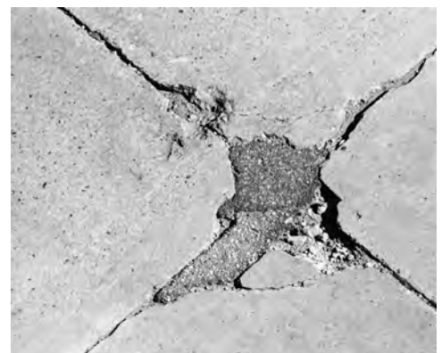
Severely spalled corner crack with missing pieces and patching.
