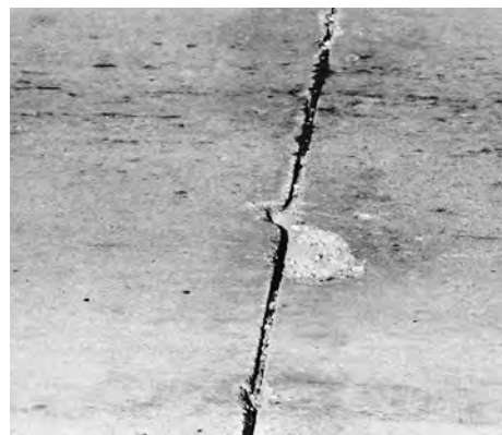
◀ Moderate spalling at transverse joint.
