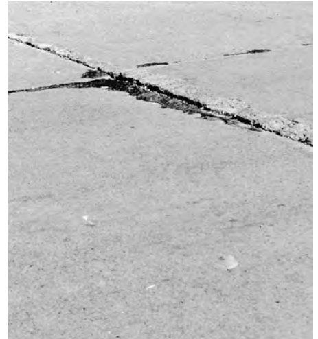
▼ Transverse joint has slight faulting and spalling.
