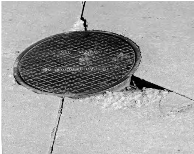
Two spalls at manhole in a new pavement. Partial depth patching would be beneficial. ◀
