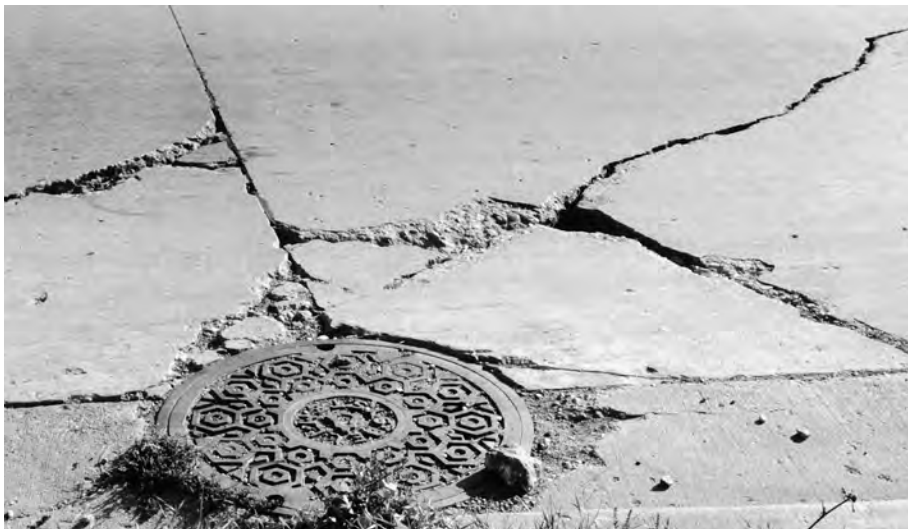
Extensive cracking and spalling at manhole requiring full depth repairs. ▼
