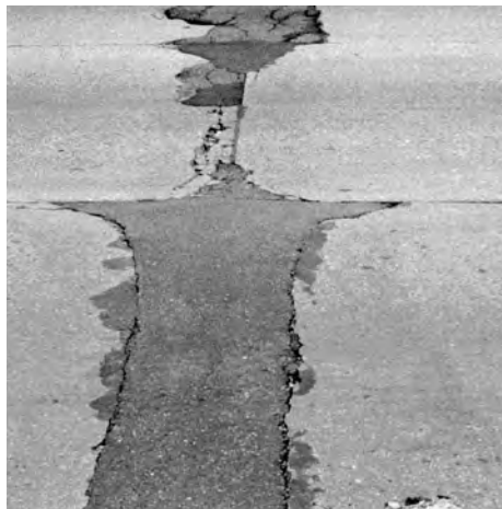
▲ Asphalt patches. Poor (top) and fair (bottom) condition.
