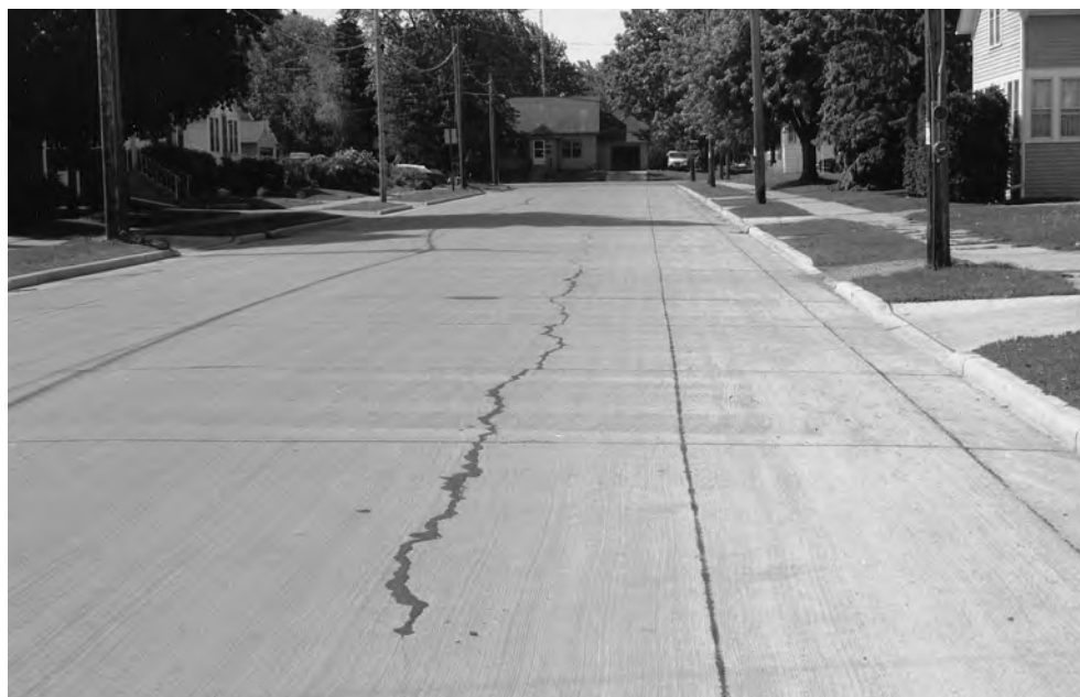
▶ Isolated meander crack, tight and well sealed.
