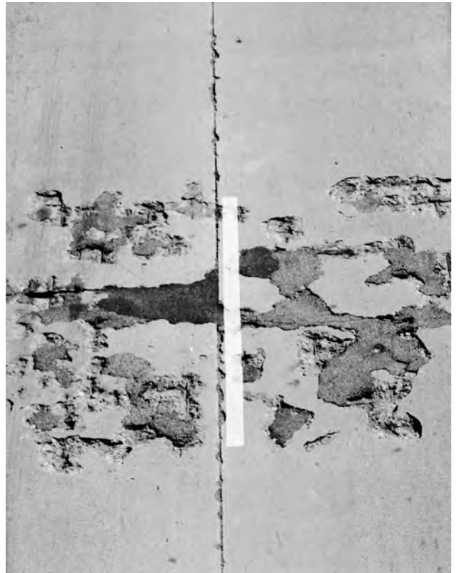
▲ Spalling caused by shallow reinforcing steel. Temporary patching needs to be followed by extensive partial depth repairs.
